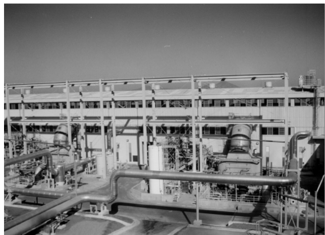
Fig.7 Spray jet condenser
