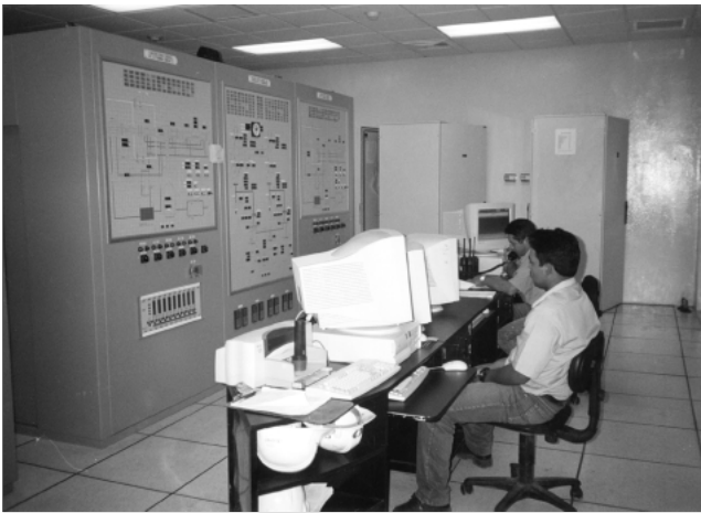
Fig.10 Plant control room
